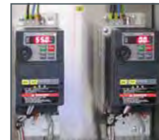
Frequency converters for controlling the pumps
