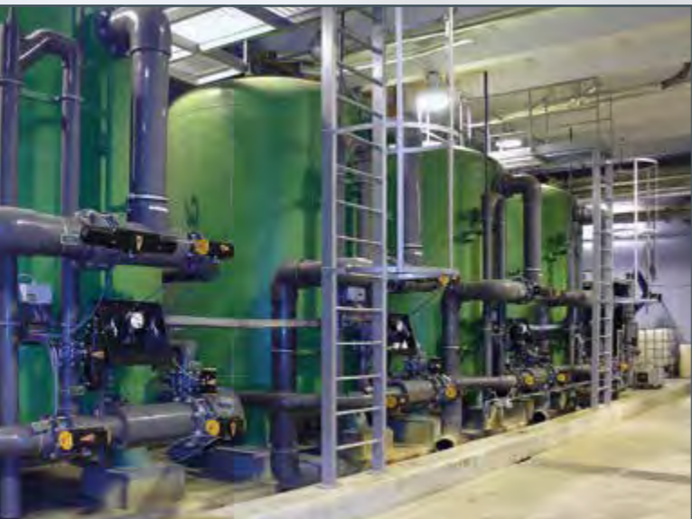
Continuous-flow adsorber in a water treatment plant
